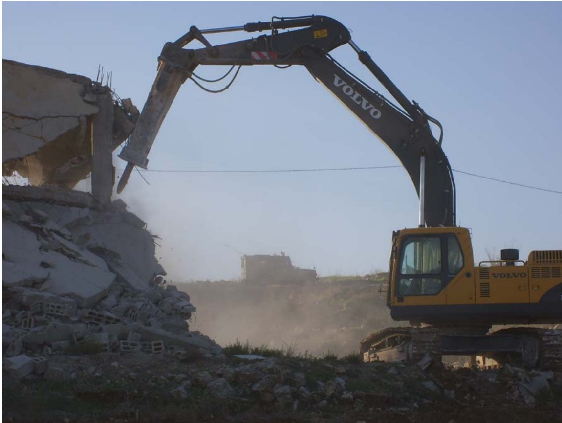
Photograph of Volvo machinery destroying Palestinian home at Hajja December 6, 2006. Courtesy, Israeli Committee Against House Demolitions
