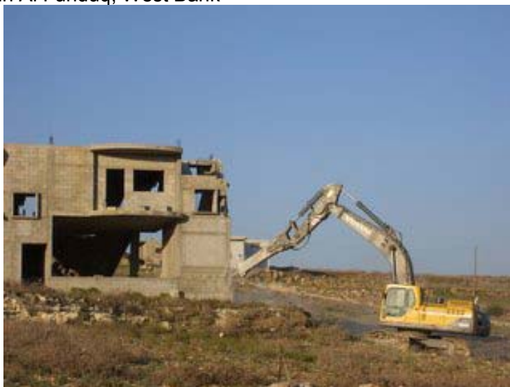
Source #10 - House Demolition Photos, Al Funduq, 22.11.06 - Caterpillar & Volvo equipment demolishing house in Al Funduq, West Bank
