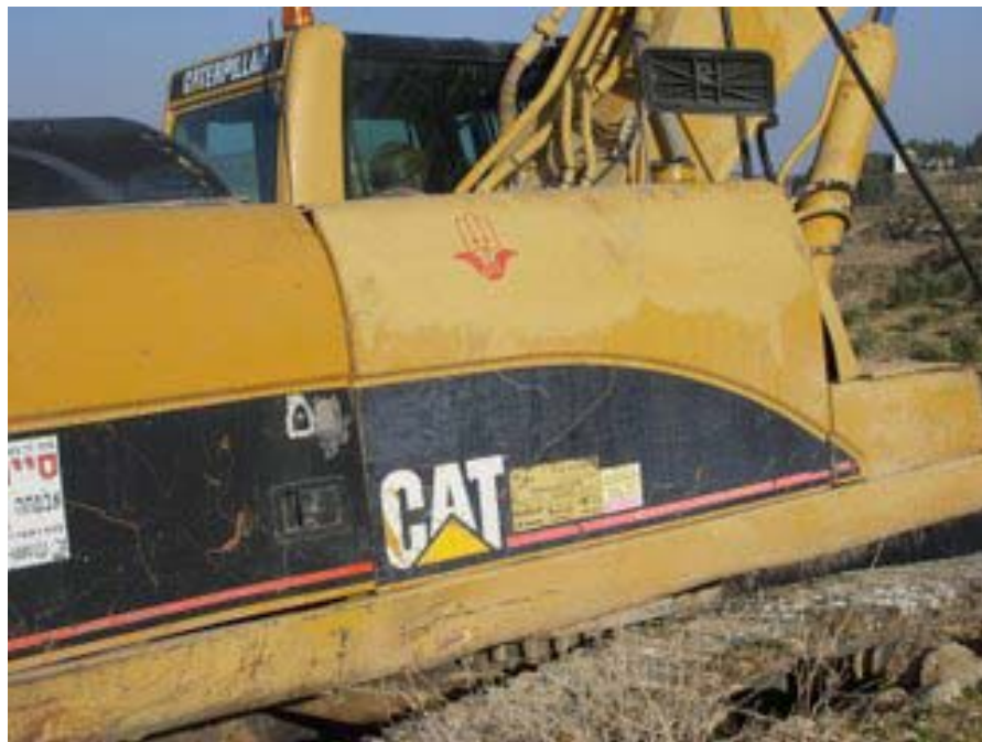
Source #4 – Photos of Caterpillar bulldozer destroying a home at Al Funduq in the West Bank
